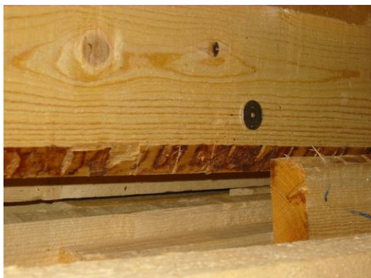
Figure1 – Wane on edge of board is not regulated.
