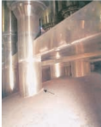
Figure 9: Deposits around the reactor head penetrations
