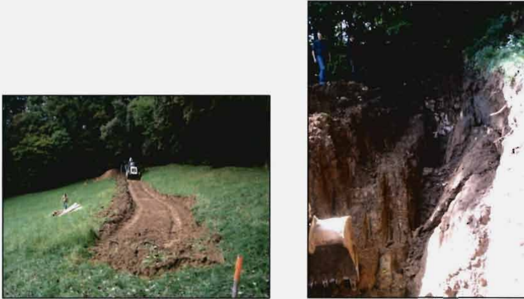
Fig. 4. Initiation of excavation in trench #1 (left) and the collapse of the wall that stopped the works (right). Note the contact of PI,Q sediments with Badenian limestone on the right picture
