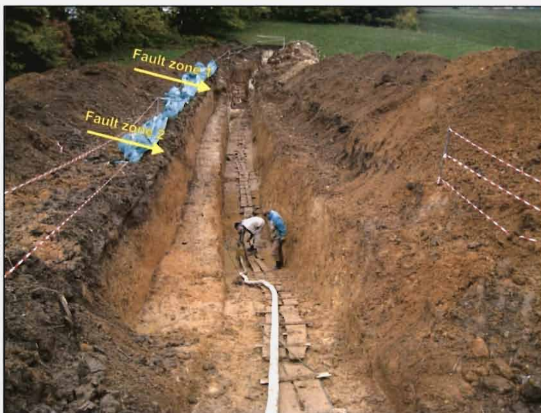
Fig.4. Trench 2 during cleaning and extraction of meteoric water. Fault zones FZ1 and FZ2 are marked.
