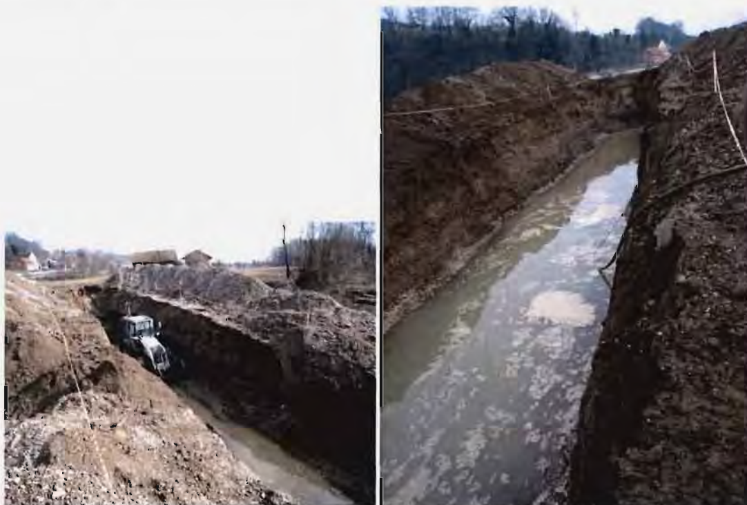
Figure 40. Groundwater inflow (app. 4 l/s) affected stability of trench wall.
