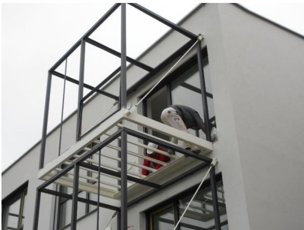
Figure 12: Unsafe performance of work at heights
