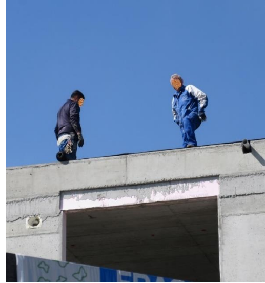
Figure 4: Non-use of personal protective equipment
