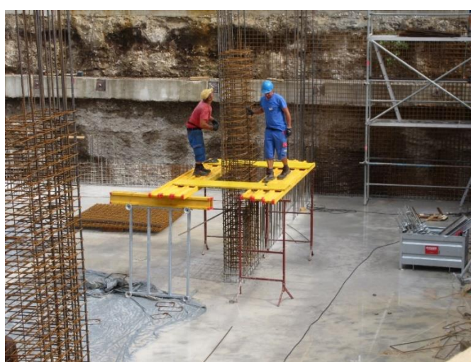
Figure 11: Unsuitable workplace – construction site improvisation
