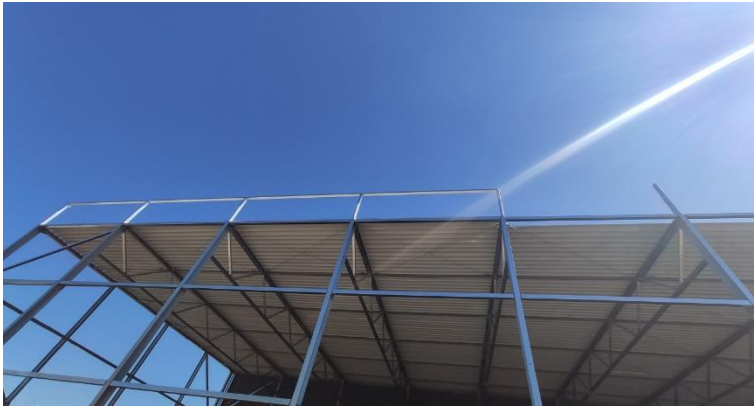
Figure 14: The place on the roof from which the worker fell
