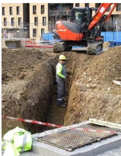
Figure 10: Unsuitable workplace – construction site improvisation
