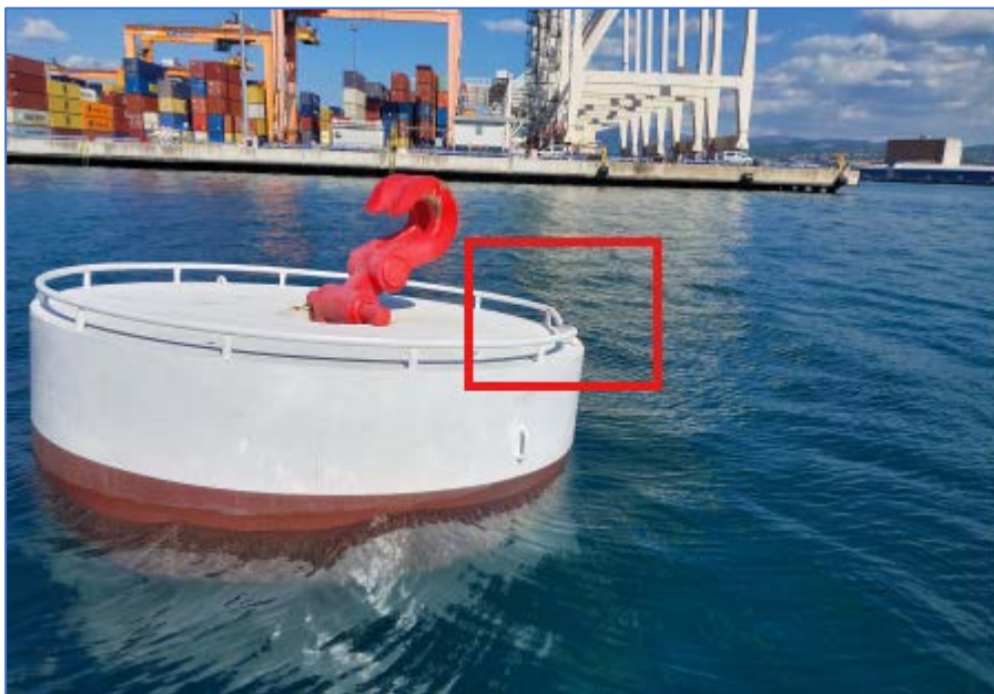
Photo of a mooring buoy; damage indicated by the red square
