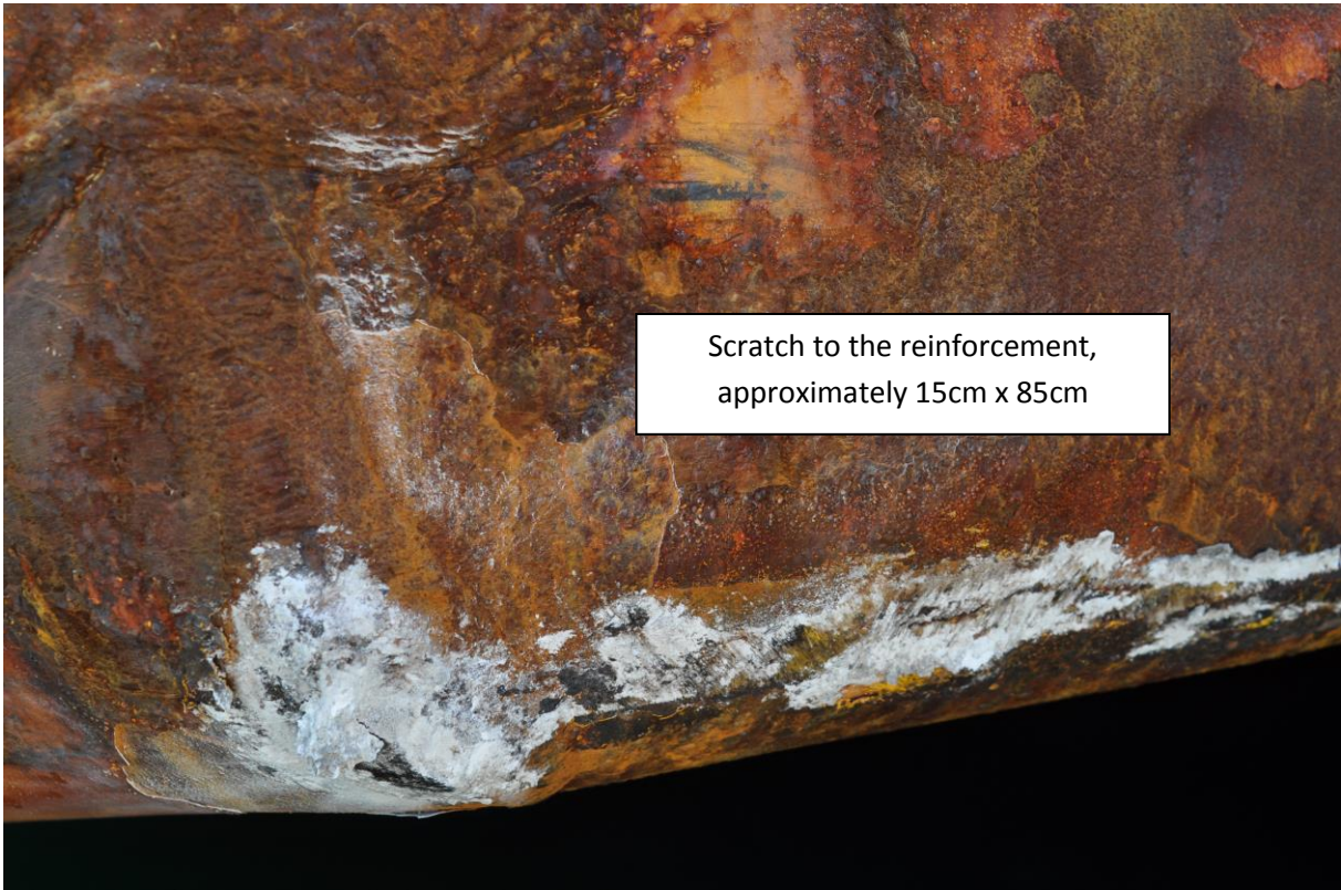
Picture 5: Damage to the reinforcement
