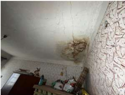
Pogled : strop v slabem stanju
