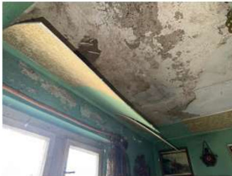
Pogled : strop v slabem stanju
